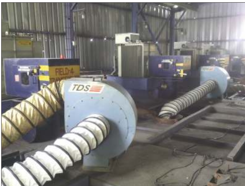
TDS installation in factory setup.
